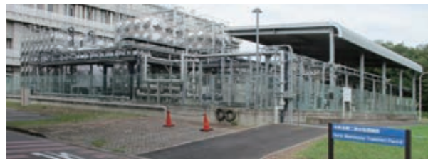
Wastewater treatment facility in AIST Tsukuba
