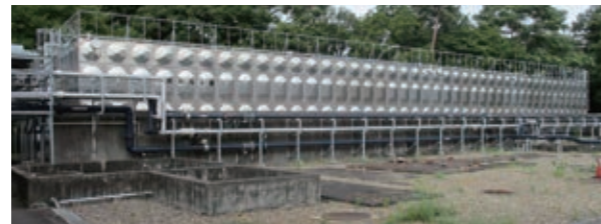
Recycled water tank in AIST Tsukuba
