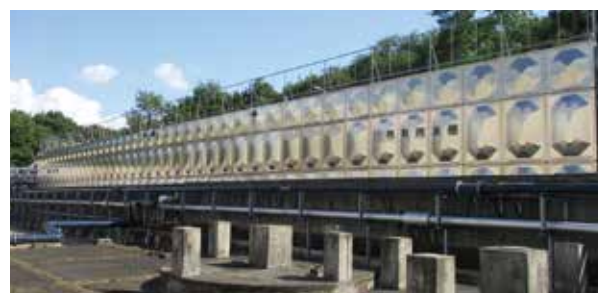
Water reuse plant at AIST Tsukuba
