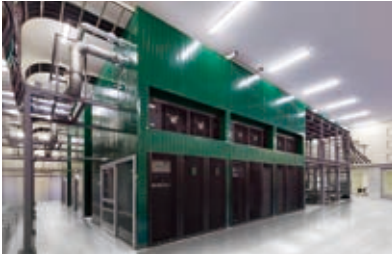
Inside a server room in the AI Data Center
