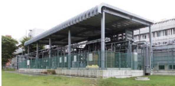
Wastewater treatment plant at AIST Tsukuba
