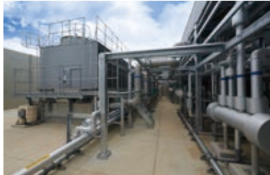
Equipment outside the AI Data Center (R: AI Data Center, L: cooling units)
