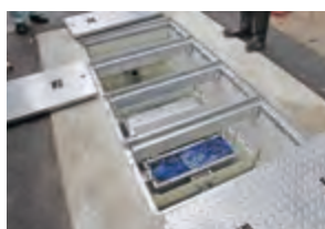
An oil-water separator installed in the kitchens at AIST Tsukuba
