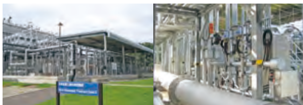
Wastewater treatment plant at AIST Tsukuba
