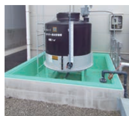
Containment bund placed around a liquid waste storage tank for exhaust cleaning equipment
