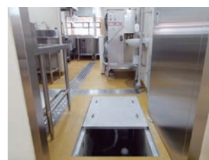
Oil-collection device connected to the grease trap
