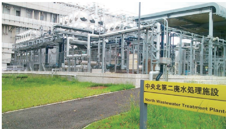
Wastewater treatment plant at AIST Tsukuba
