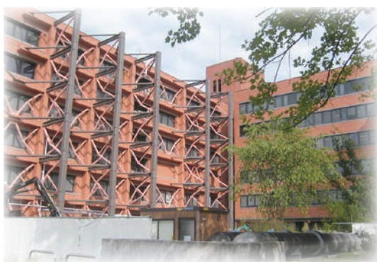
Toggle brace damper method (AIST Tsukuba Central Building 5-2)
