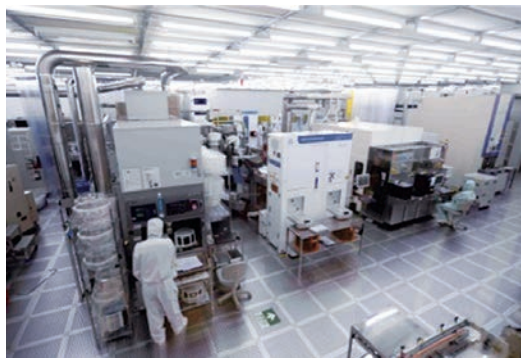
Super Clean Room
