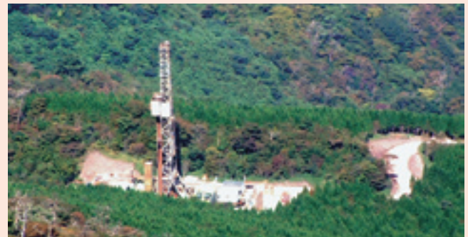
Photo Unzen Scientific Drilling site on the north-side slope of Unzen. Fifty meter-high rig were set up in an area of approximately 2000 m 2 , and a road was constructed in the national forest. (Pictures provided by Professor Setsuya Nakada, Univ. Tokyo)
