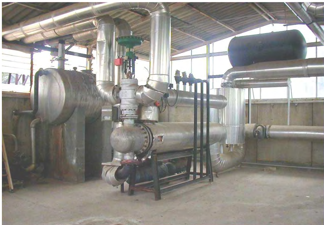
Green houses Heater
