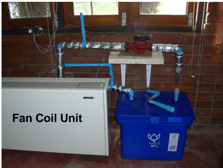
Room for Cooling (Cool Water Circulation and Fan Coil Unit)
