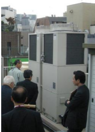
Ground source and air source hybrid heat pump
